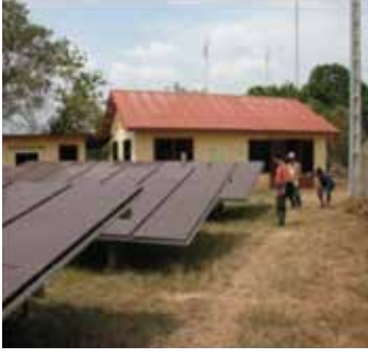
Distributed Solar Plant
