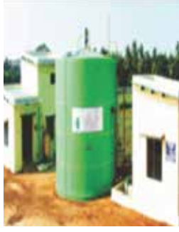
Distributed Biogas Plant
